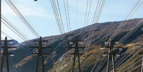
Power Line Monitoring
