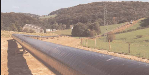
Oil and Gas Pipeline Monitoring
