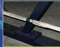
Optical Ground Wire (OPGW)
