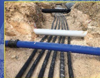
Underground Power Line Monitoring
