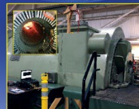
Gas Generator Monitoring
