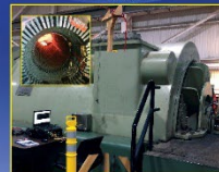
Gas Generator Monitoring
