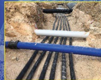
Underground Power Line Monitoring
