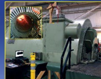
Gas Generator Monitoring
