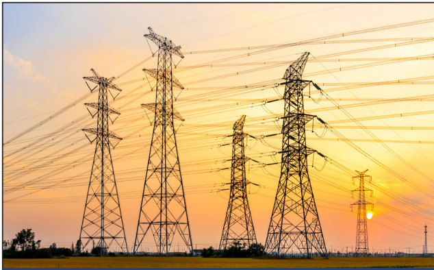
Overhead Power Line Monitoring
