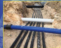
Underground Power Line Monitoring
