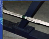
Optical Ground Wire (OPGW)
