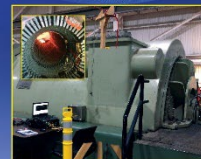
Gas Generator Monitoring
